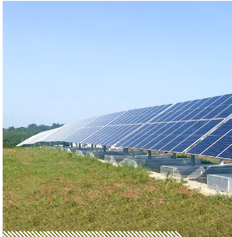
SOLAR ARRAY ON THE PORTLAND LANDFILL • Photo by ReVision Energy
