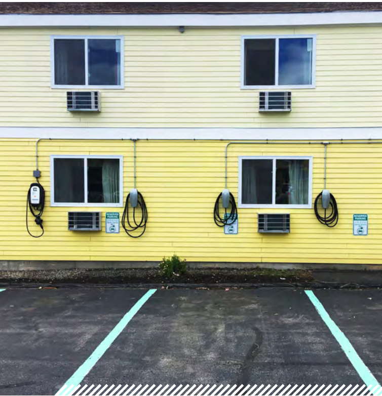
EV CHARGING AT THE SOUTH PORTLAND DAYS INN • Photo by ReVision Energy
